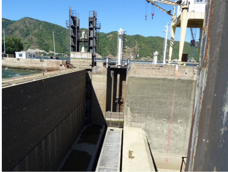
Figure 3.8 - Navigational lock "Djerdap I", upper head, overhaul-repair (in operational position) and main operational door (in the niche)
