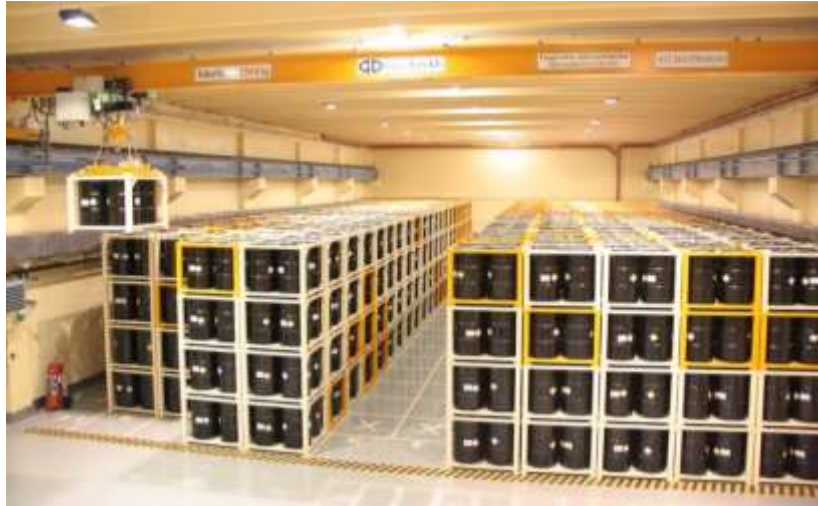
Figure 12: Technological storage of radioactive wastes in the surface facility of the NRWDF
