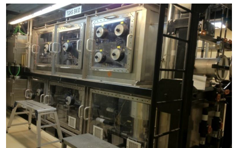
Fig. III.5-6 Tritium gas handling and storage system at WTRF-Korea
