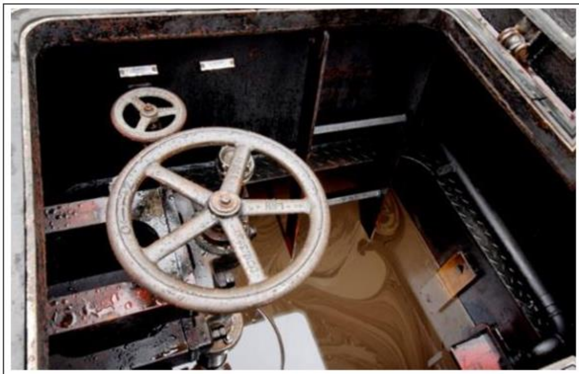
Picture No. 24: Bilge water in the hut of the vessel
