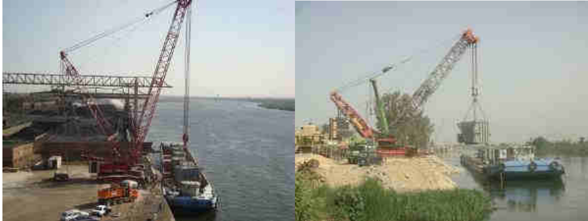
Figure 4.2. Transshipment of a transformer from the river barge on Nile (Egypt) (mass of the transformer about 150 tons)
